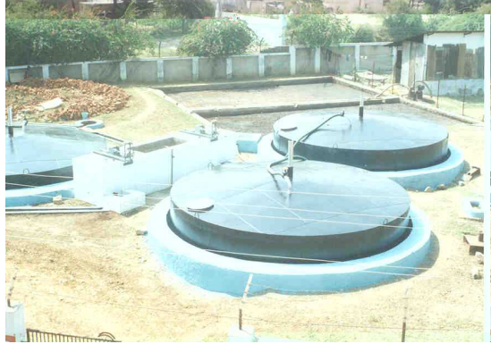
Institutional Biogas Plant(4x85 cub. m.) at Dakor temple committee, Gaushala
